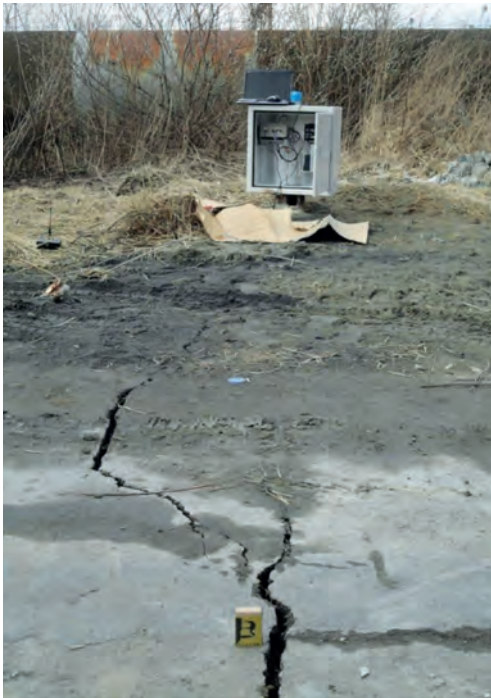
Fig. 4. Crack on the ground surface resulting from the backfill of the space beyond the lining
