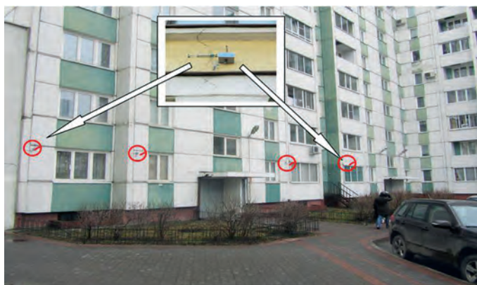
Fig. 5. Location of the instrumental monitoring sensors on the façade of one of the buildings
